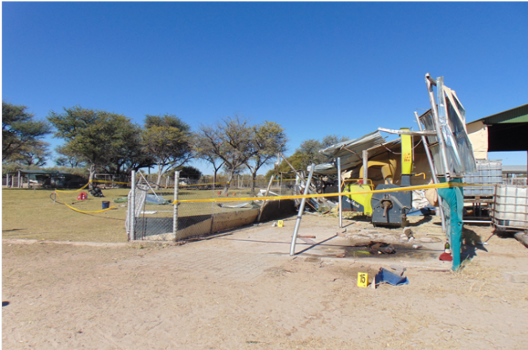
Figure 2b: Front view of the decimated roof of the milling shed next to the main farm shed.
