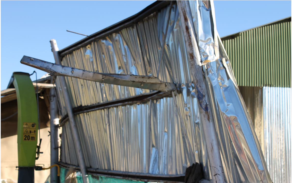
Figure 2c: View of the roof beam structure that probably caused the aircraft to flip over.
