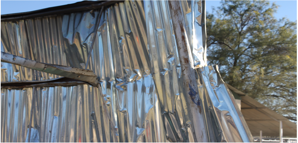
Figure 2: View of the next collision impact point after the vehicle shade which is a milling equipment roof next to the farm shed.
