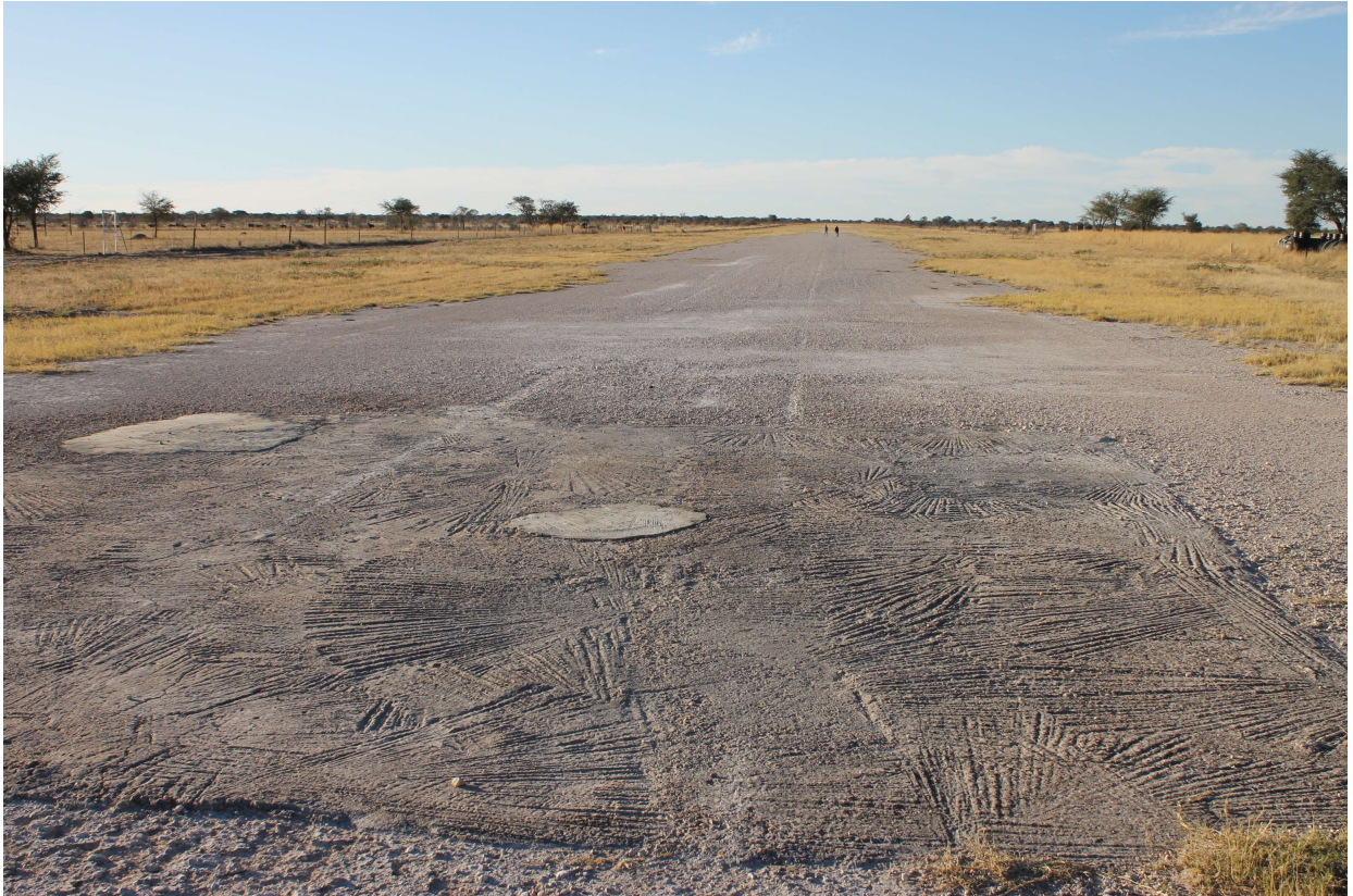
Figure 6: view of the main gear tracks over the engine run-up area.
