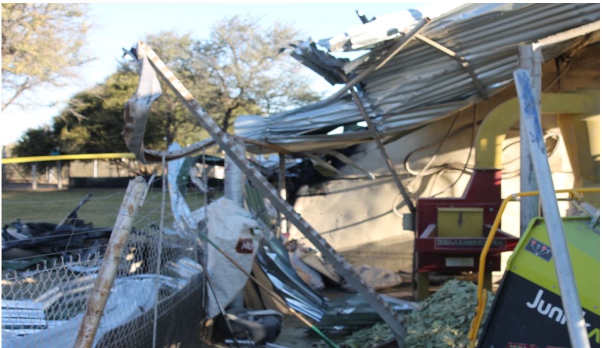
Figure 2d: The decimated roof truss of the milling equipment structure.
