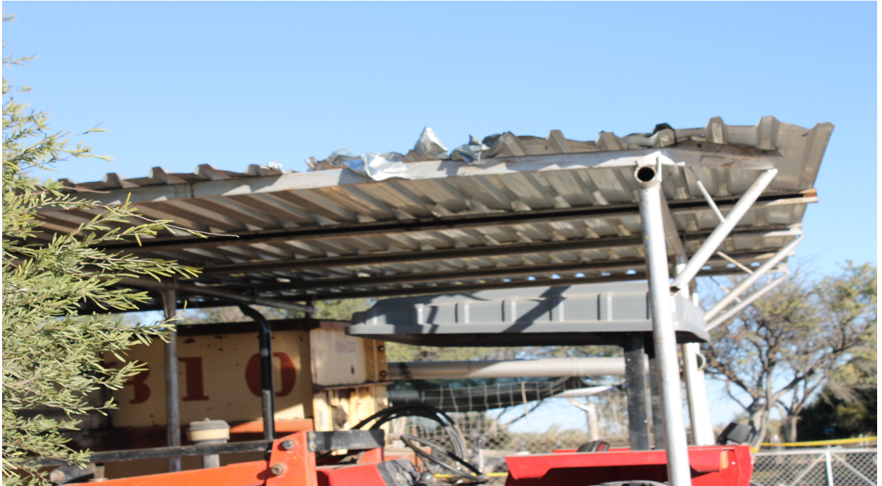
Figure 1c: Close view of the resulting damage on the vehicle shade roof structure
